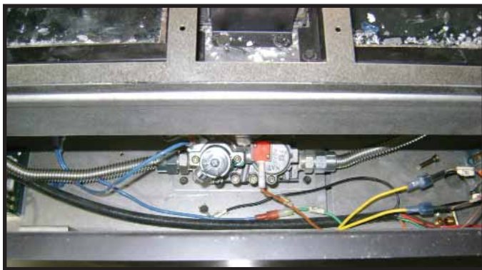
Figure 11.1. Valve Pressure Taps.
